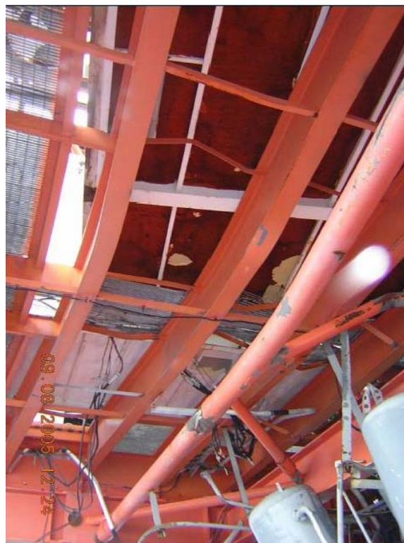
FIGURE 6. MAJOR DAMAGE TO DECK STRUCTURE DUE TO WAVE IMPACT
