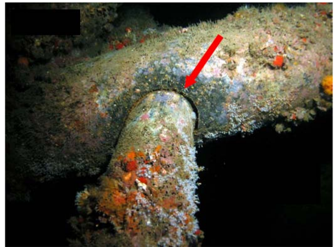
FIGURE 4 – DAMAGED T JOINT DUE TO INADEQUATE JOINT CAN THICKNESS
