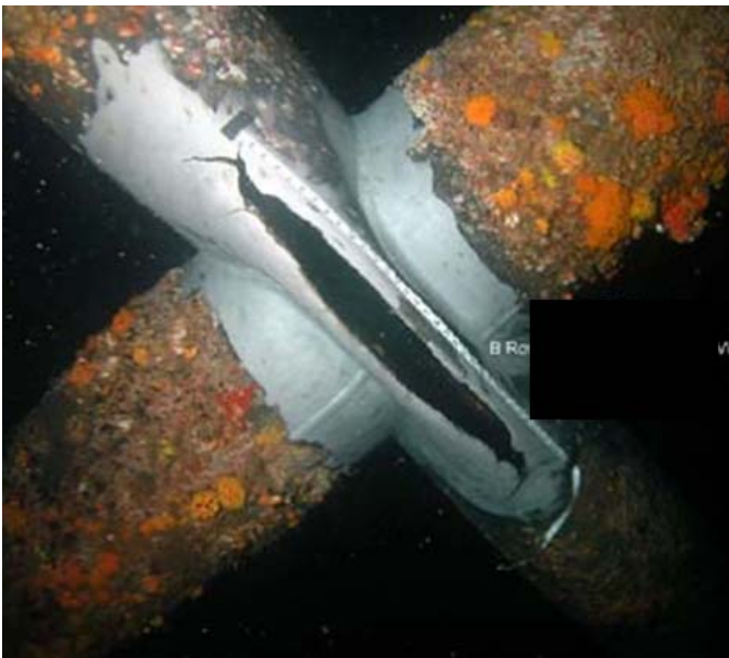
FIGURE 3 – DAMAGED X JOINT DUE TO INADEQUATE JOINT CAN THICKNESS
