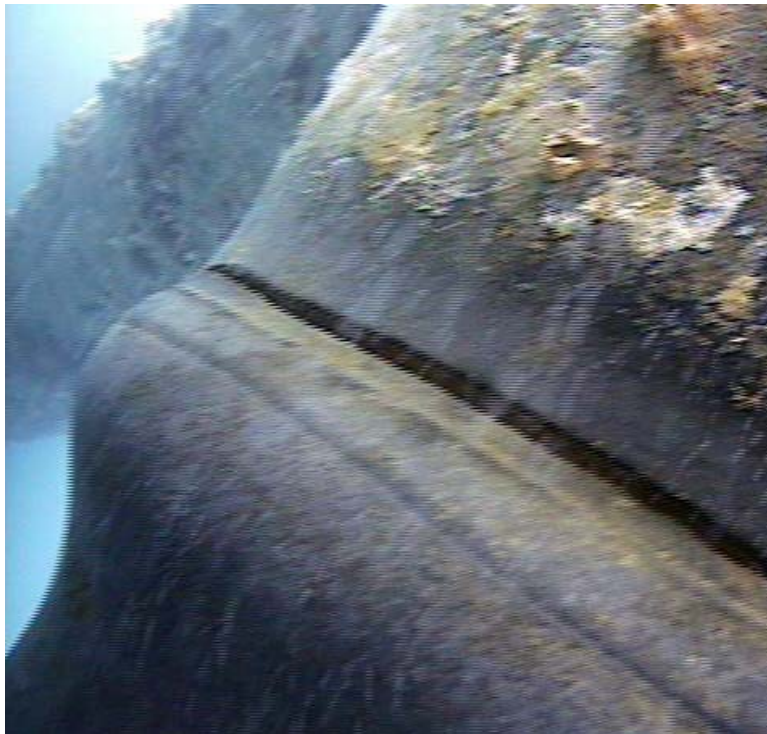
Figure 6: Severed leg section just above the bulge. Note the longitudinal weld seam just below the sever.
